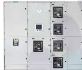
MCC Control Panel
