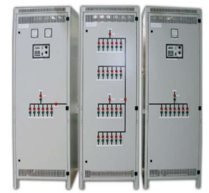
AC & DC Drive Panel
